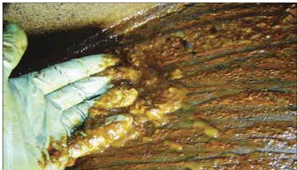
Figure 1. Sludge on Reservoir (Courtesy of Clarus Technologies).
