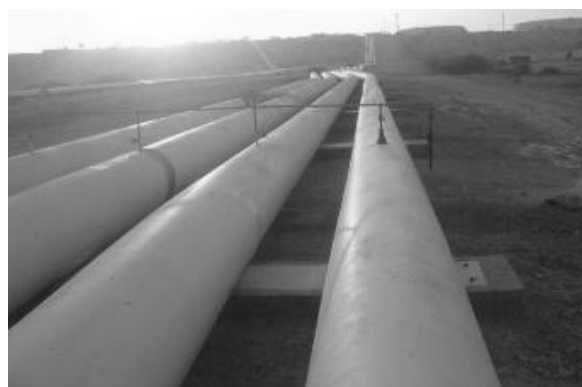
Figure 2. The Kharg oil pipeline under investigation.
